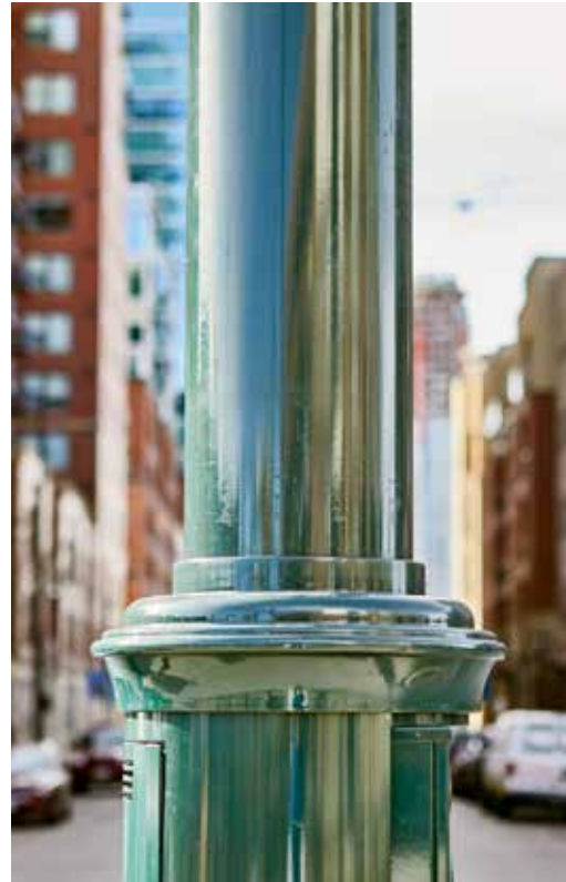
Architectural shroud between base cabinet and upper pole.
