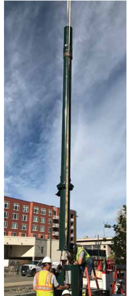
Step 3: Install top section with antenna onto base section with architectural shrouds.
